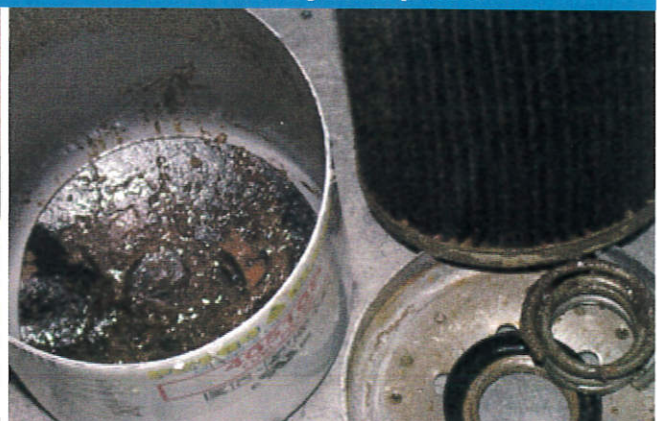
F3. - Corroded Dispenser Filter
