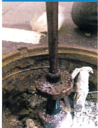
F1. - ATG Floats w Corrosion Products
